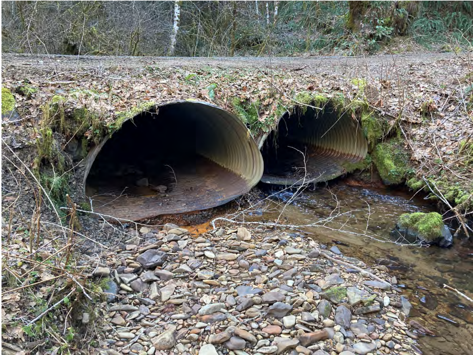
Swartz Creek mainstem: downstream of culvert 2/23/2023
